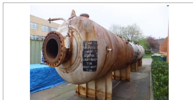
Condensate flash separator vessel used for the case study
